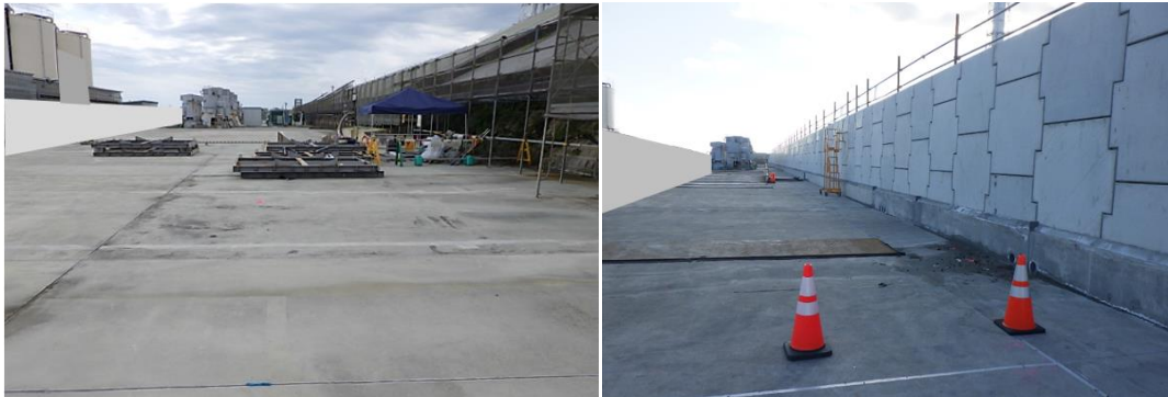
Installation work for the Japan Trench Tsunami seawall (left: before, right: after)
