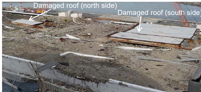
Status of the roof on the Unit 3 turbine building [Before start of construction] [Shot taken from the west side]
