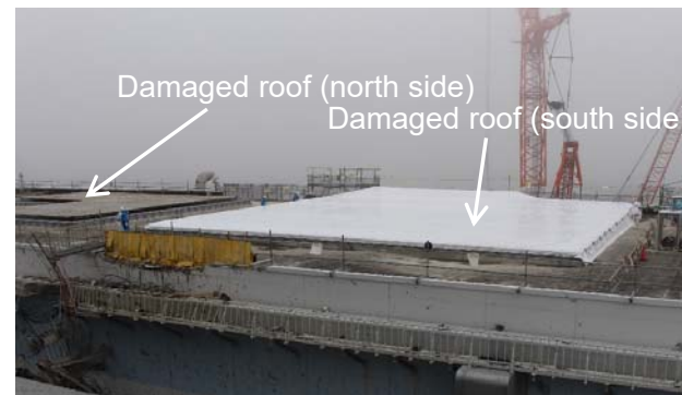
Status of the roof on the Unit 3 turbine building [Completed installing the discharge prevention weir/rainwater cover (south side)] [Shot taken from the west side]
