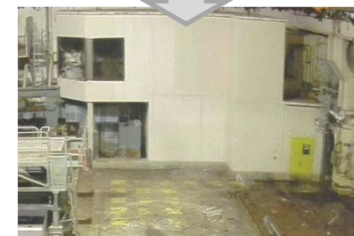
Before and after removing the residual items on the Unit 2 refueling floor
