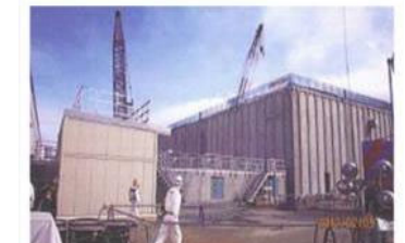
Temporary waste sludge storage
