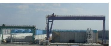
Spent adsorption vessel temporary storage facility
