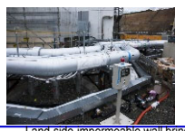
Sub-drain purification system
