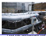
Sub-drain purification system
