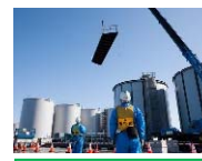
Land-side impermeable wall brine (refrigerant) circulation pipe
