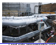
Sub-drain purification system
