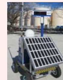
Installation of Dose-rate monitor
