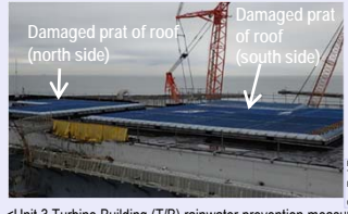
<Unit 3 Turbine Building (T/B) rainwater prevention measures> In August 2020, installation of the rainwater cover completed
