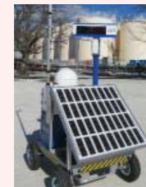
Installation of Dose-rate monitor
