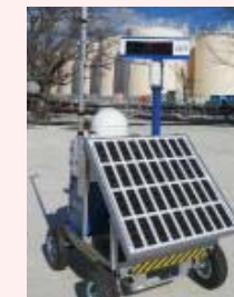
Installation of Dose-rate monitor
