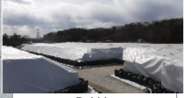
Rubble (outdoor accumulation)
