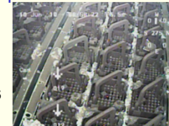
The upper part of fuel assemblies and fuel racks
