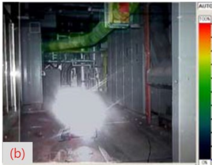
Figure 3.2.3 Gamma camera photo of the southeast area of the 1st floor (2) (December 2013) [6]
