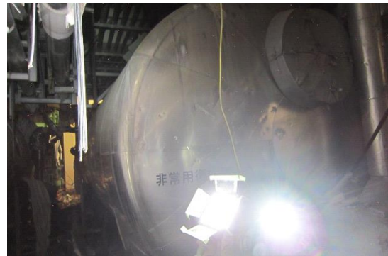
(B) IC tank north side
