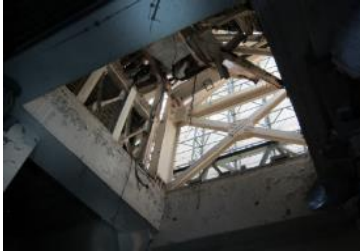
Figure 7 Equipment hatch after hydrogen explosion (view from Floor 4 to Floor 5)
