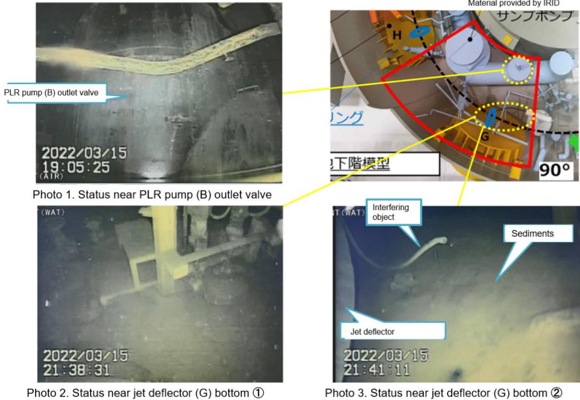
Figure 2-57 Status near the PLR pump (B) and near the jet deflector (G) [2-32]
