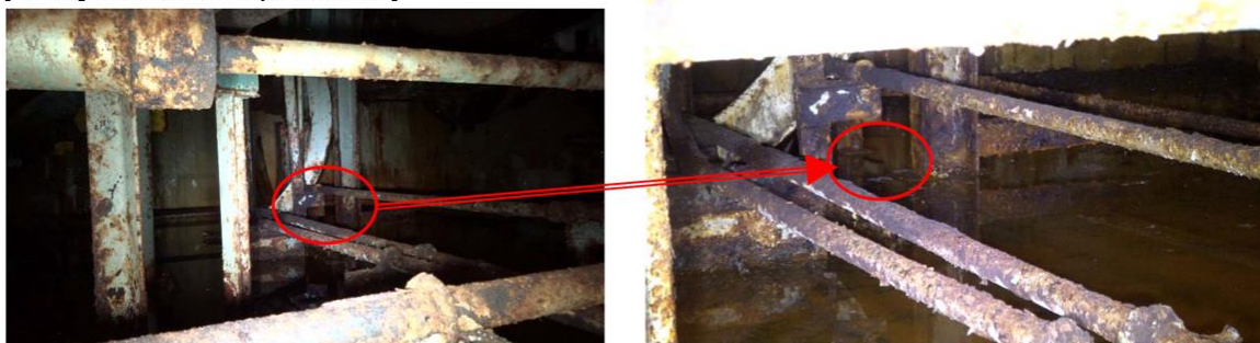
Main steam piping D (at the rear of main steam piping C)
