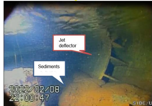
Sediments near jet deflector ④
