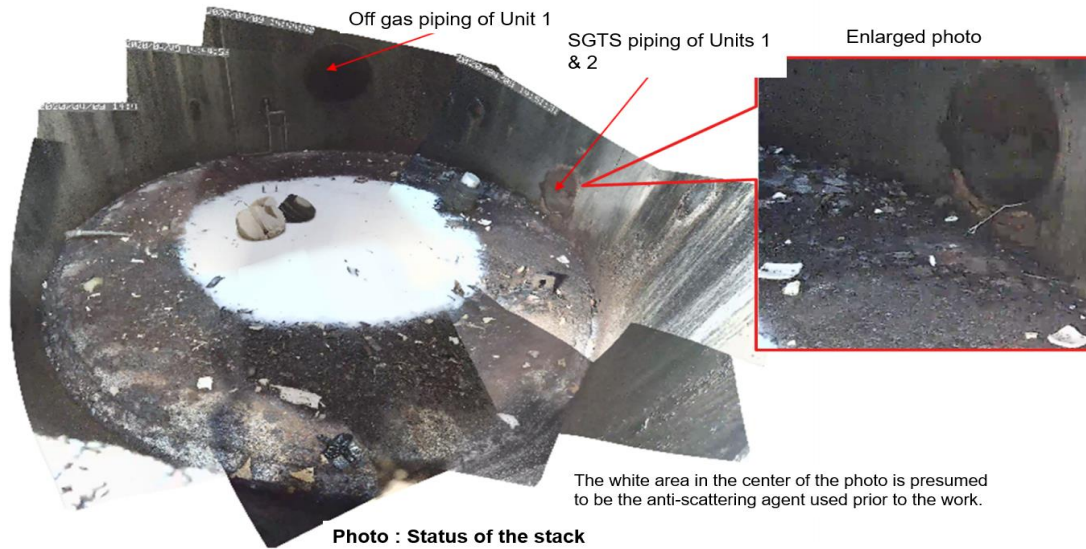
Figure 2-42 Condition at the bottom of the exhaust stack [2-25]
