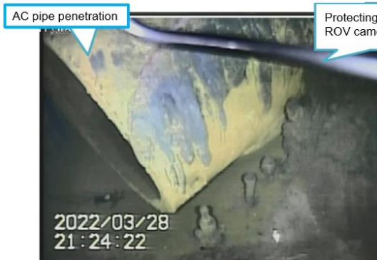
Photo 2. Status of AC pipe penetration
