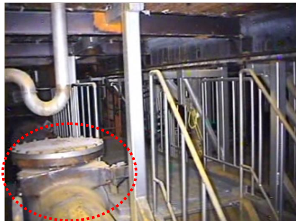
Figure 2-3 Photo of an S/C vacuum breaker in the torus room of Unit-1 (part)
