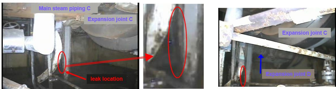
Main steam piping D (at the rear of main steam piping C) Enlargement of leak location
