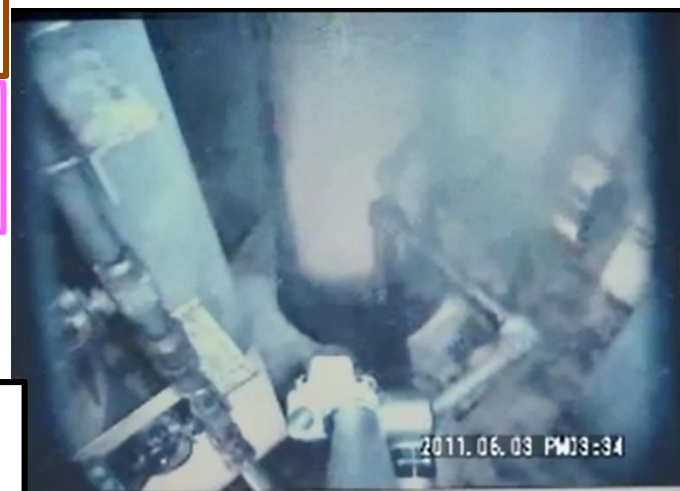
Steam observed at a floor penetration in the southeast area (June 2011 photo)
