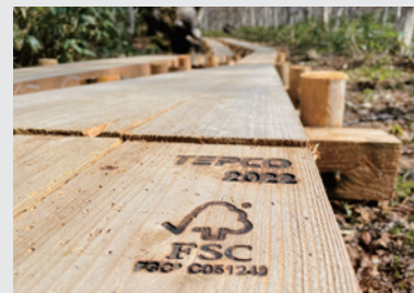
Leveraging the Oze Tokura Forest (FSC certification) By using lumber to repair the wooden path, we are fixing CO 2 , and promoting transport cost reductions through local-production/local-consumption.
