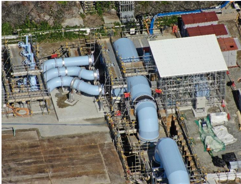
Seawater transfer pipes and seawater header pipe (Header pipe: ALPS treated water is mixed and diluted with seawater) [photo taken on June 25, 2023]
