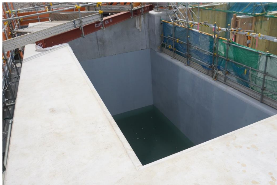
Discharge vertical shaft (down-stream storage) after it has been filled with water [photo taken on June 6, 2023]
