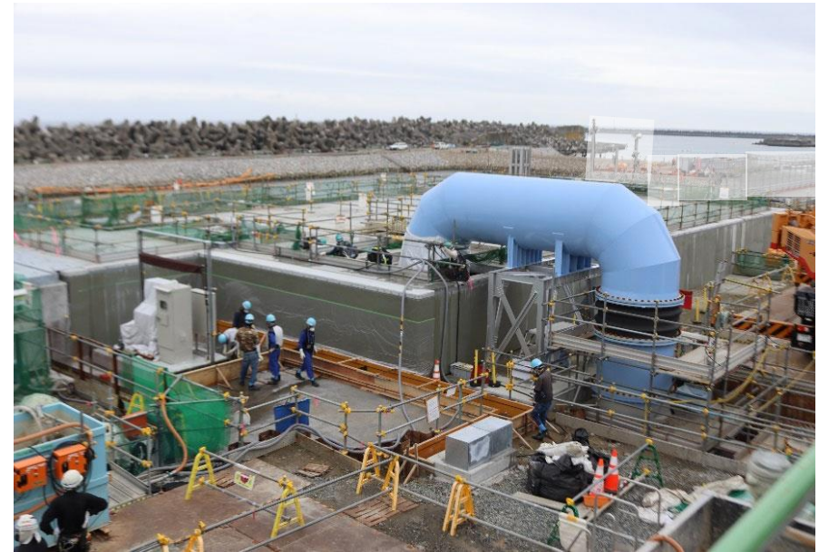
Discharge vertical shaft (upper-stream storage) [photo taken on June 23, 2023]
