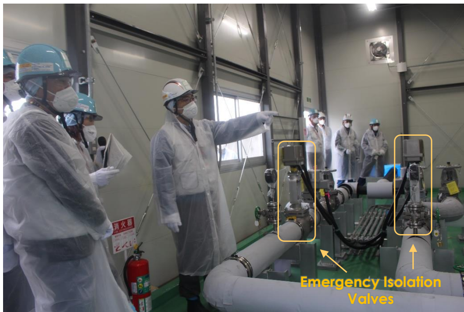
Inspection of emergency isolation valves by the International Atomic Energy Agency (IAEA) [photo taken on June 2, 2023]
