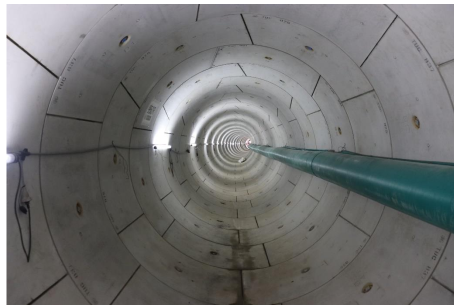
Inside of the discharge tunnel after excavation [photo taken on May 23, 2023] (The lights and the air ventilation duct were removed prior to discharge)
