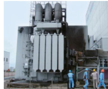
Fire at the Unit 3 house transformer
