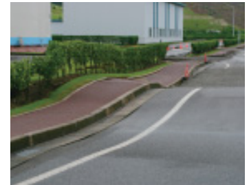
Buckling in the road shows the scale of the earthquake
