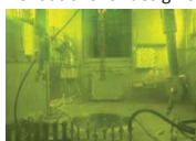
Hot cell general view
