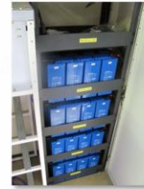
Cell Site Backup Batteries (source: Vodafone)
