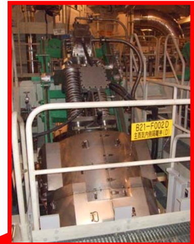
主蒸気隔離弁(8台)
