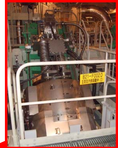
主蒸気隔離弁(8台)
