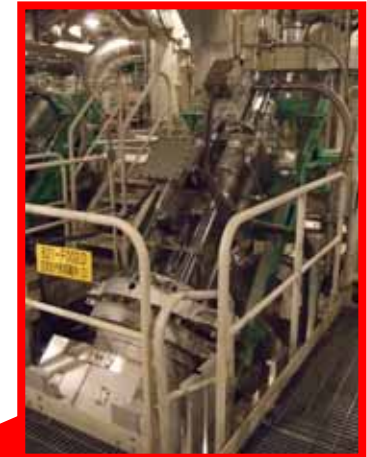
主蒸気隔離弁(8台)
